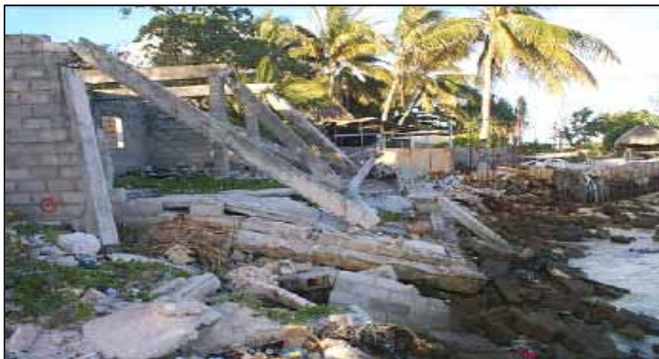
Where inappropriate development changes natural coastal processes erosion can result in property loss and huge expense in protection measures which are often unsuccessful.
